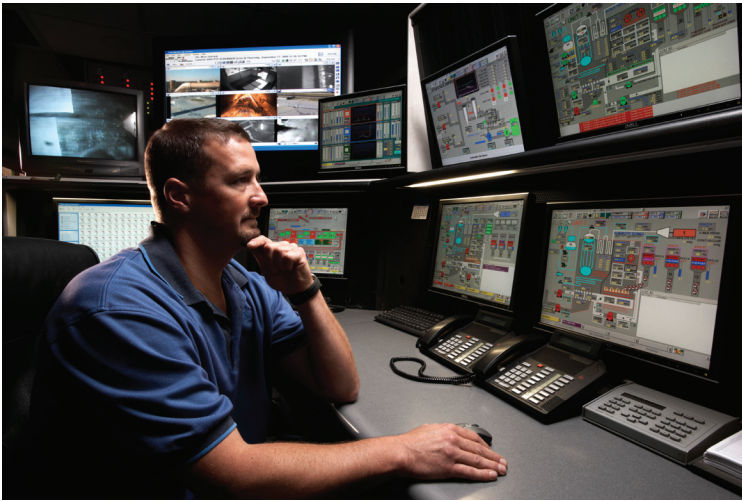
Figure 2 - Keeping tabs on the equipment's condition from the control room at Elk River Station.
